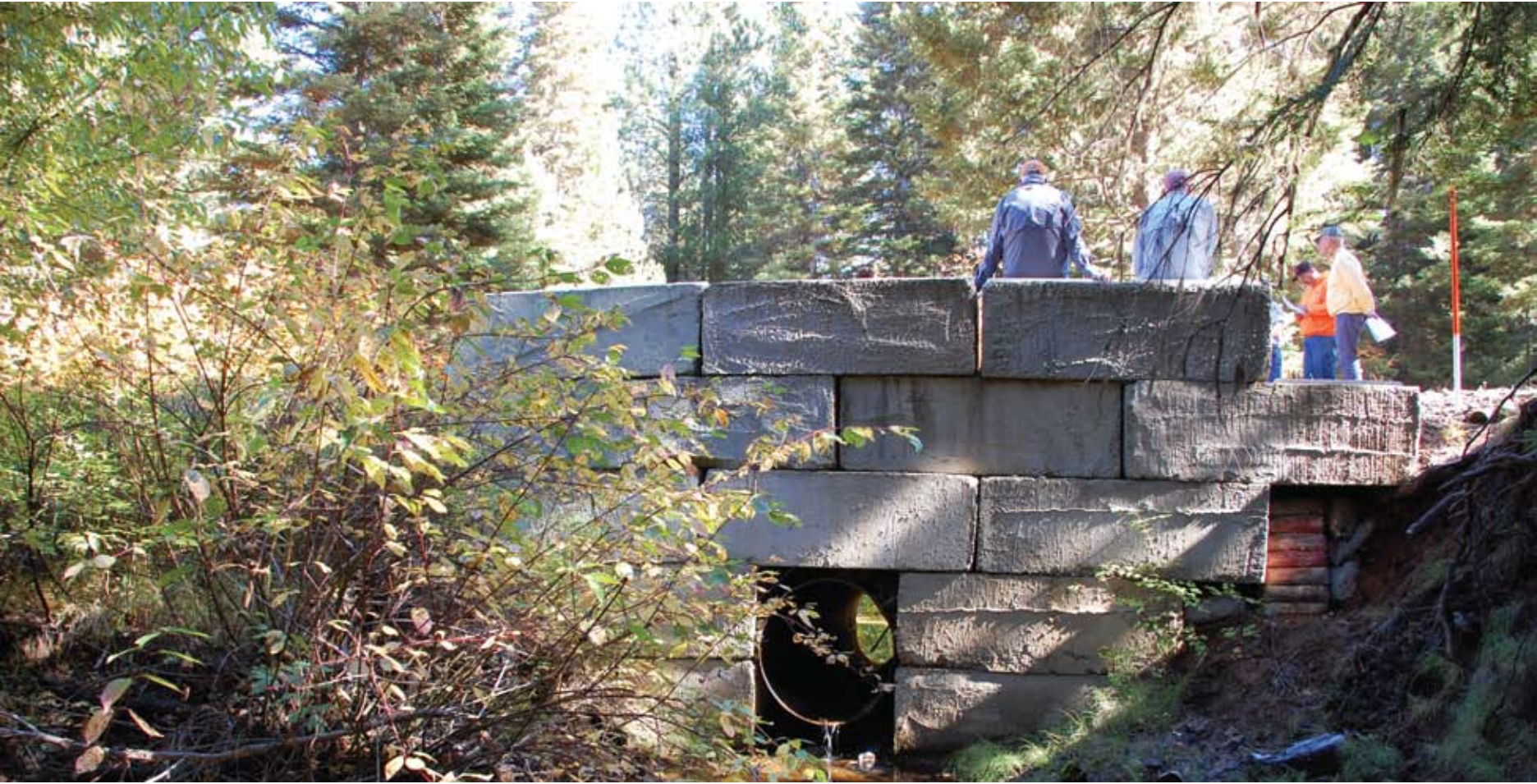
Before photograph of the culvert on Wagon Wheel Road in the Teanaway.
