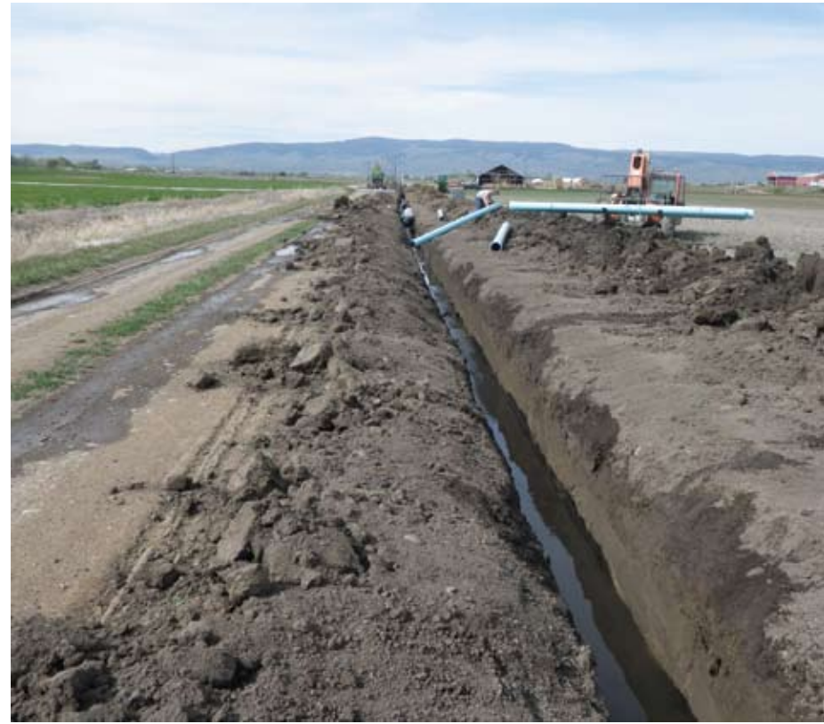
Installation of the mainline for a new linear sprinkler system northwest of Ellensburg.
