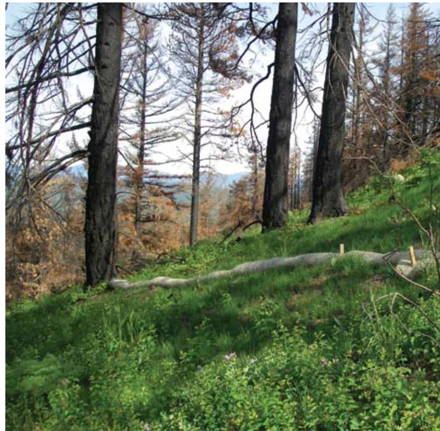
Vegetation is beginning to recover along Hart Road. Straw wattles were placed along steep slopes to help control erosion.
